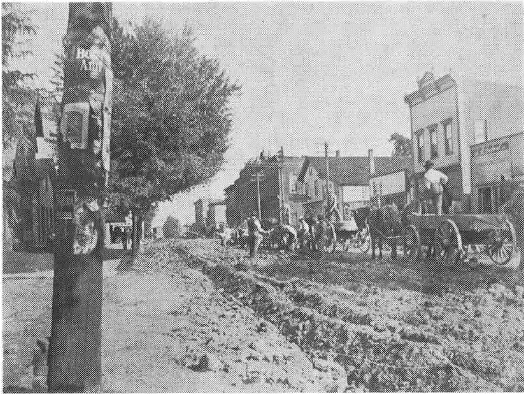
PAVING WEST MARKET STREET—Crews dug up the roadbed in 1898 to replace the dirt, dust and cinders with bricks. Dump wagons were used to haul away the top layer of earth after it had been loosened and crumbled by plowing. Picture was taken from the North Vine Street intersection at about the spot now occupied by Henderson's Sobio Service Station.
